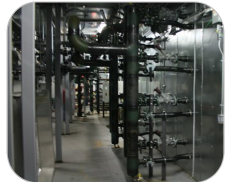
Using Quickpen, TMI modeled the piping for this unit, minimizing the amount of piping and maximizing the amount of clearance.
